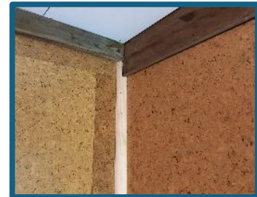
The skirting in the top corners
