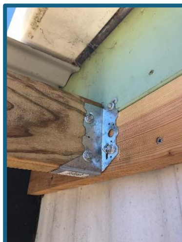
Attaching the roof beams to the exterior wall of the jam room
