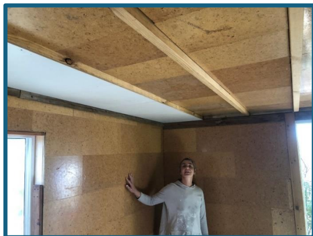
Mum admiring the clad control room
